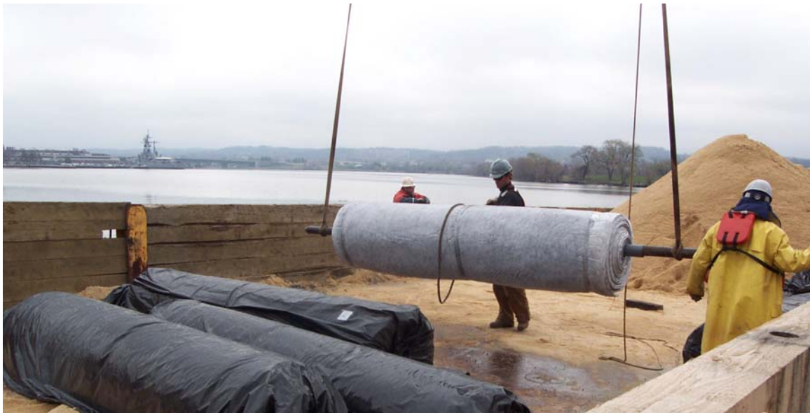
FIGURE 2. Reactive material mat being deployed at the Anacostia River Demonstration Project, Washington DC.
