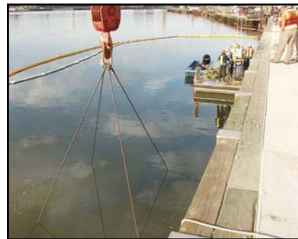
The mattress system's subaqueous installation is aided by divers to ensure proper positioning of the mattress sections.
