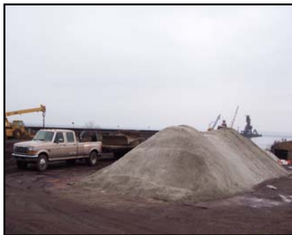
Bulk Organoclay® was used to absorb the NAPL from the affected groundwater.
