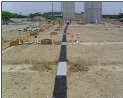
Liquid Boot® GeoVent trenchless gas venting system installation directly on the sub-grade.
