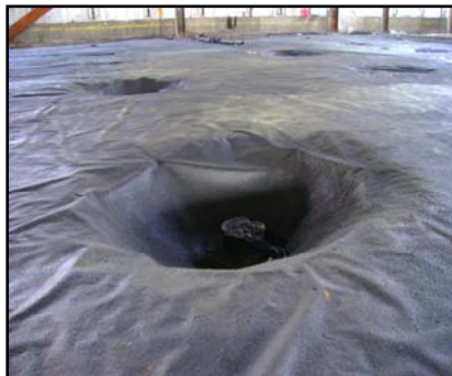
The installed spray-applied gas vapor membrane attaching to the piles themselves and conforming to the haunch.
