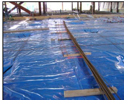
Other trade installations commencing on top of completed membrane, which has been covered with a protection layer.
