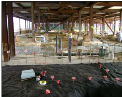
Completed gas vapor membrane (foreground) and other sections (background) due to receive membrane in following phases of construction.
