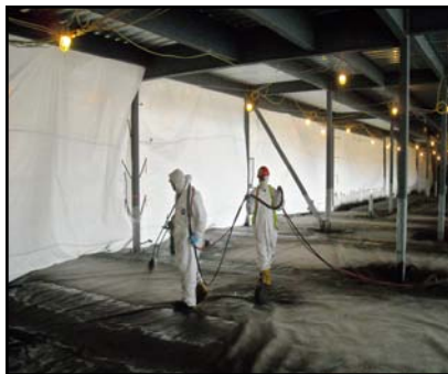
The spray-application allows for quick and air-tight seal around all penetrations and irregularities, saving considerable time and money.
