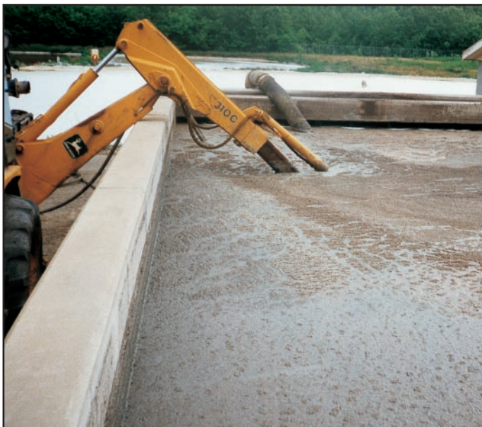
Tannery Sludge before dewatering
