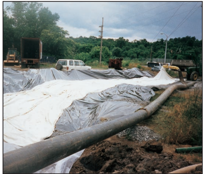
Empty GEOTEX® Tubes are spread throughout graded area in preparation for filling.
