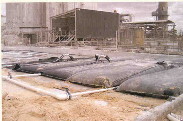
Photo 1. The switch to woven geotextile bags for sludge solids removal enabled secondary conditioning to begin after two weeks when previously the facility operators had to wait up to six months.
